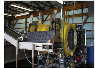
The City Sewer Plant's new sludge rotary machine, shown above, was put into service in mid-July.
